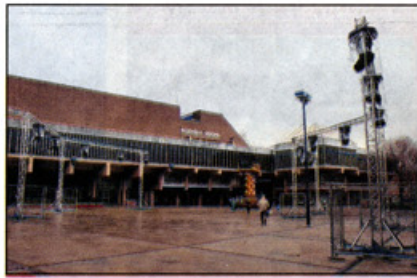
LET THERE BE LIGHT: The gantries for the lights and projectors are erected in Derby's Market Place ahead of the start of the Under Scan project tomorrow. Picture: Maria Marshall MM220206B-1
